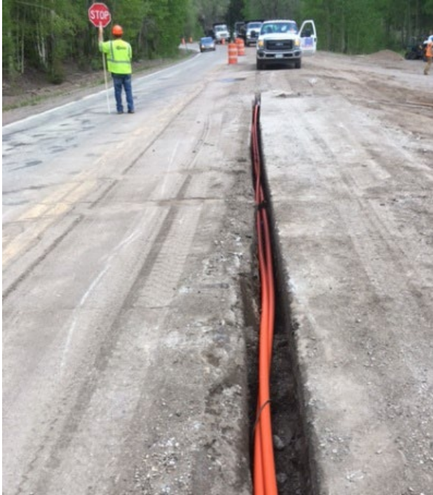
Figure 4: Colorado Department of Transportation installation of fiber optic cable during a mill and overlay project
